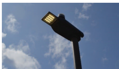
Figure 22: Axia 3 new street light units have been installed in the AONB (by Urbis Schreder)
